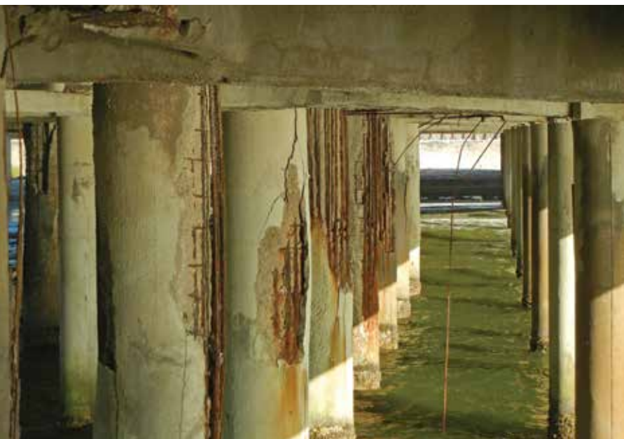
Fig. 1: Deteriorated columns between water line and deck
